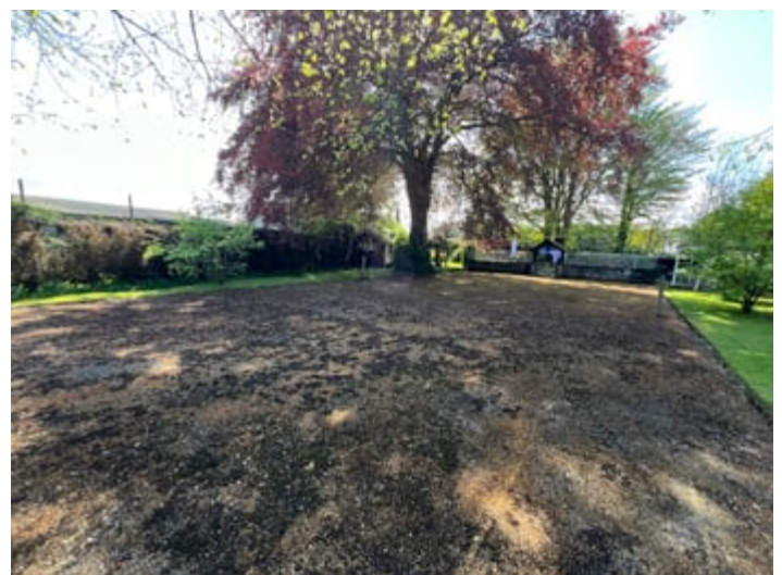
Which offers a full sized court being tarmaced, this court is in need of re-surfacing.
