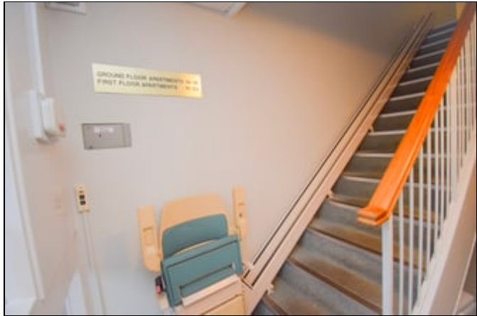
Stairs up to first floor with stair lift, automatic lighting, storage heater.
