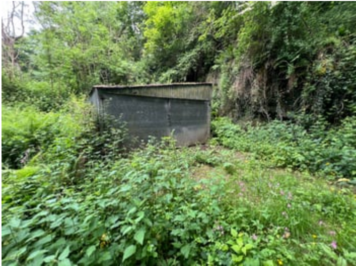
20' 0" x 14' 0" (6.10m x 4.27m) of timber construction with zinc sheets and steel double doors.
