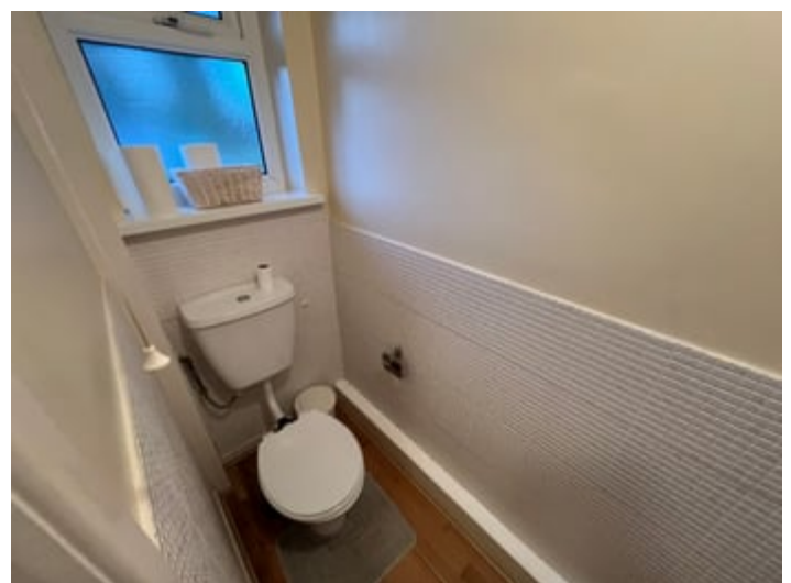
With dual flush w.c. enclosed shower unit with Heatstore electric shower above, half tiled walls, frosted window to rear, Dimplex radiator.
