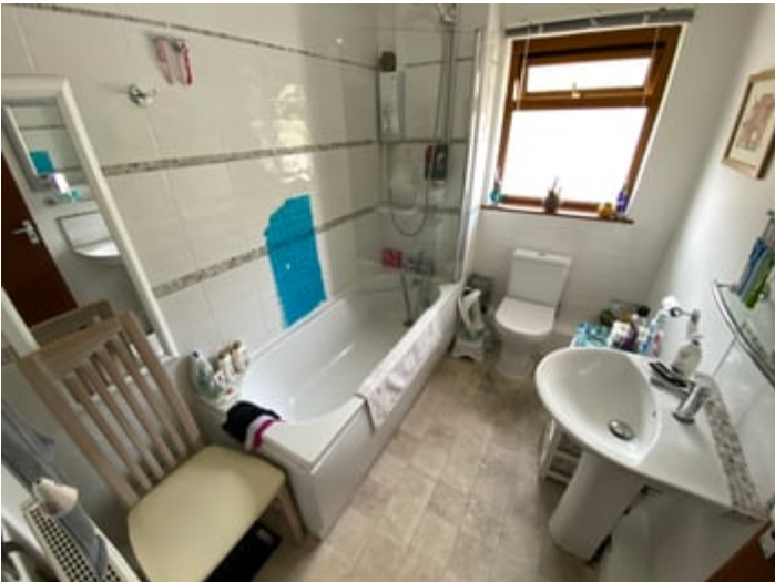
8' 7" x 6' 2" (2.62m x 1.88m). A modern suite with a panelled bath having shower over, low level flush w.c., pedestal wash hand basin, extractor fan, radiator.
